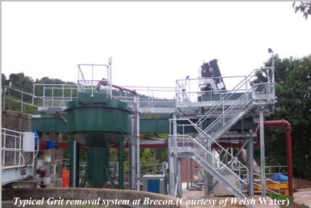
Typical Grit removal system at Brecon. (Courtesy of Welsh Water)
